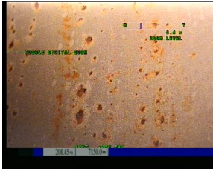
Figure 8. Discontinuities on the inner surface of the reactor pressure vessel.
