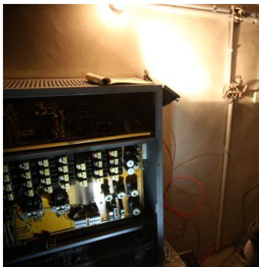
Picture 2: Relay controller frequently used
