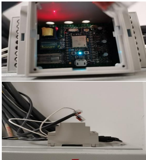
Fig. 4. General view of the IoT smart electricity meter
