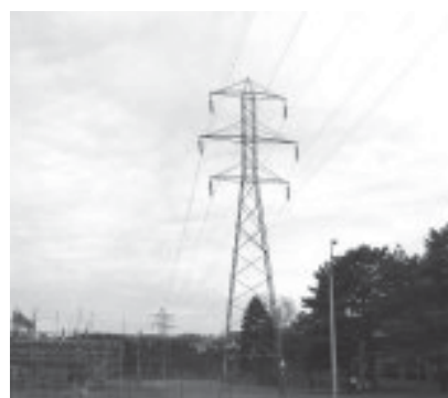
Fig.2. 2x110 kV three-phase power line.
