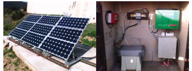
Fig. 3. The grid connected PV system.
