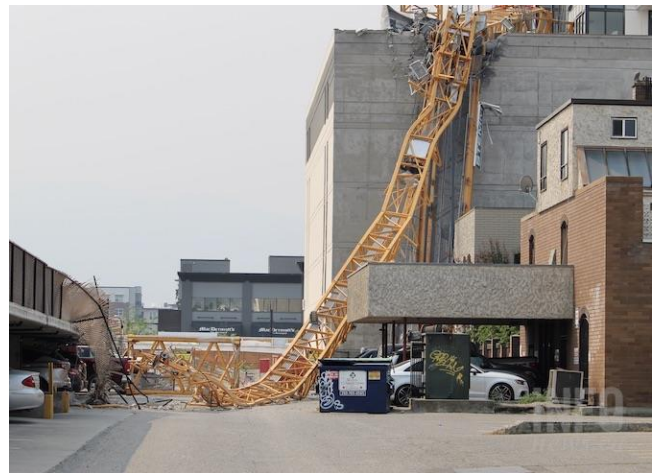
Fig. 1. Buckling failure of tower crane
